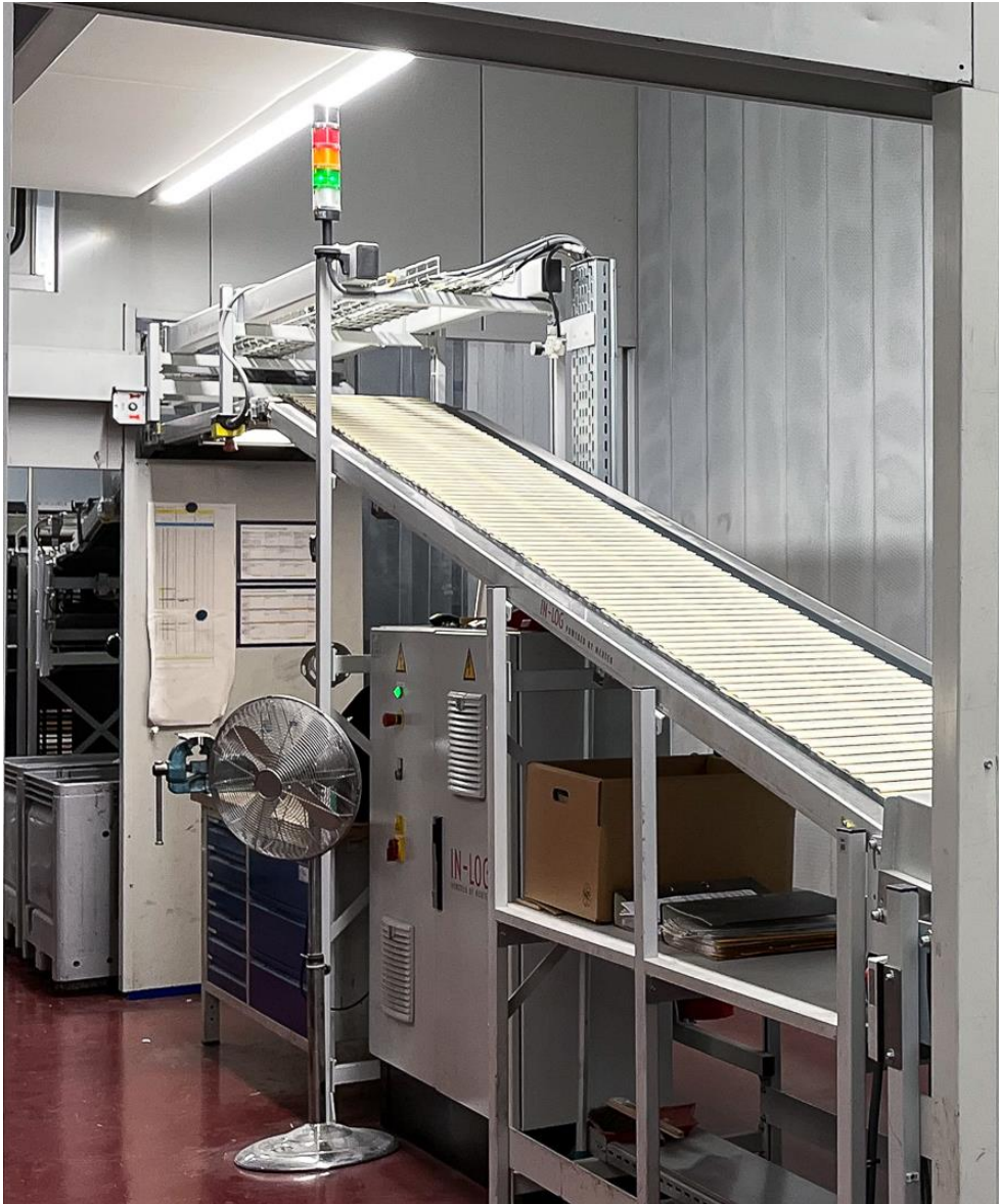
▲ The space underneath the high conveying section has been used to place the electrical control cabinet.
